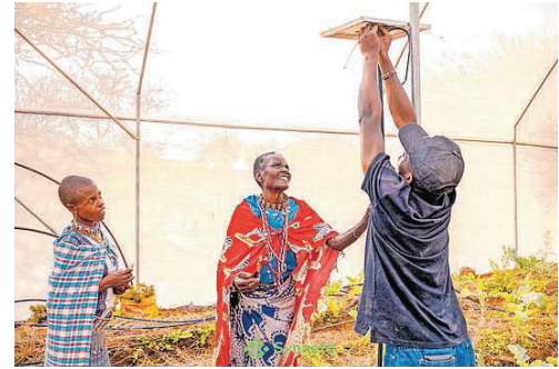
A Synnefa technician, Daniel Nduati, installs a solar panel to power a farm. PHOTO | EDDY ASHIOYA
