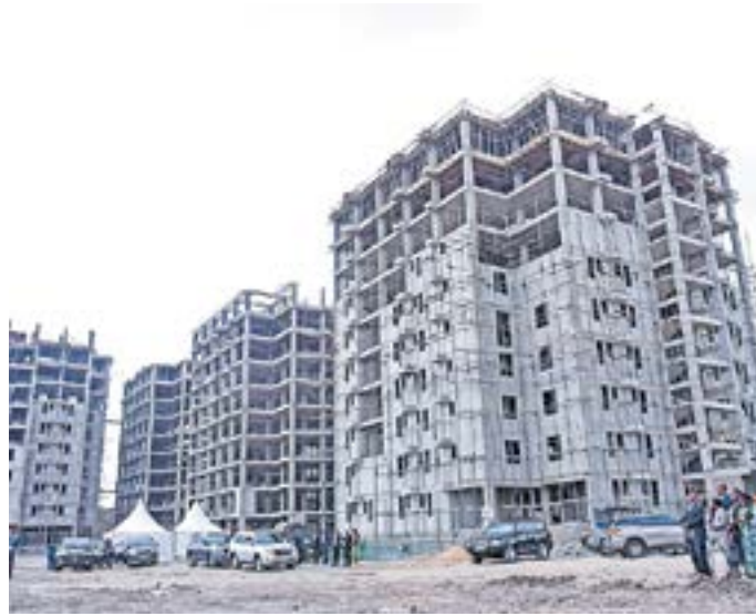
An affordable housing project in South B, Nairobi. EVANS HABIL I NATION
